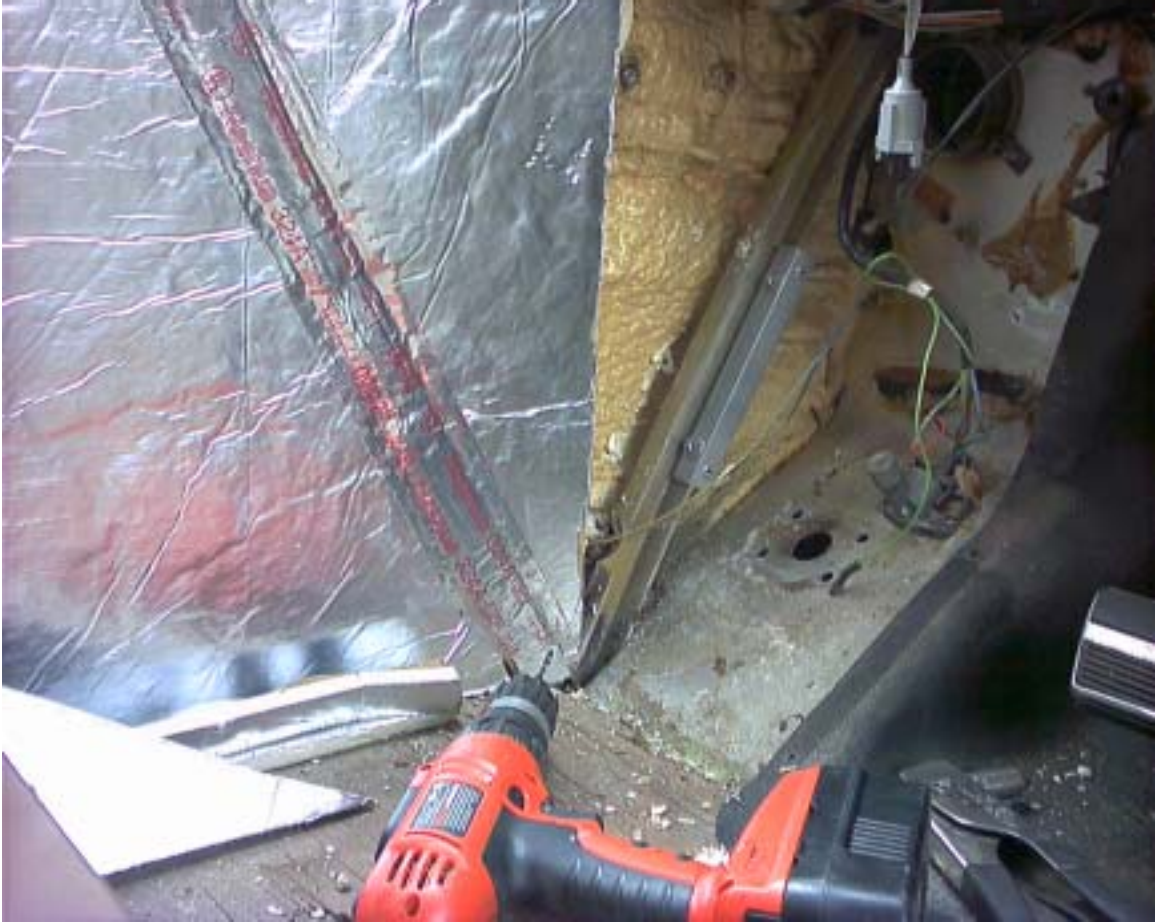
The Aluminum angle bracket provides a fastening point for the new FRP kick panel.
