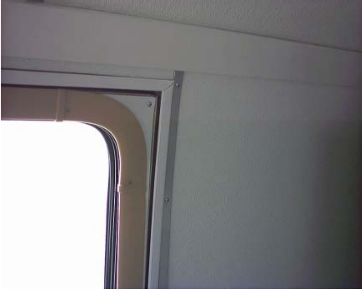
The new door molding fit like a glove and looks good against the new wall panels.
