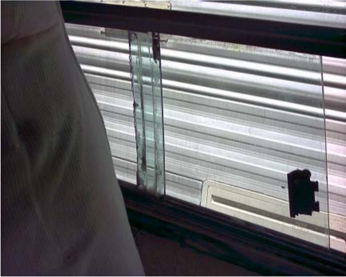
Adhesive had been used to retain the vertical bar in addition to the screws.
